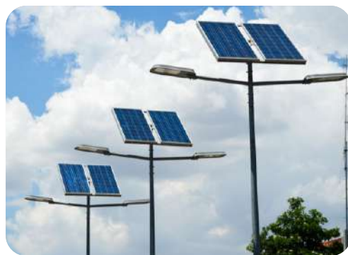
Solar Street Light
